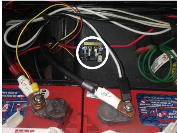
Figure 19. Photograph of where current sensor, circled, is mounted.
